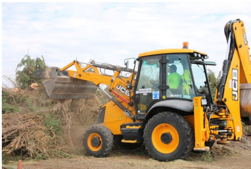
Image above: Backhoe at the Wodonga RRC pushing up the garden waste pile
