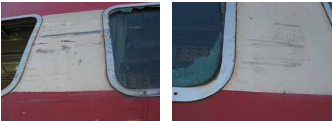
Figure 9. Initial scuff mark forward of the second window (right) progressing to window frame notch and gouging (left).
