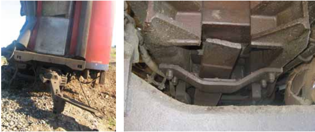
Figure 21. Fractured draft yoke at site, forward end of BN19 (left) and rear of BRN20 (right).
