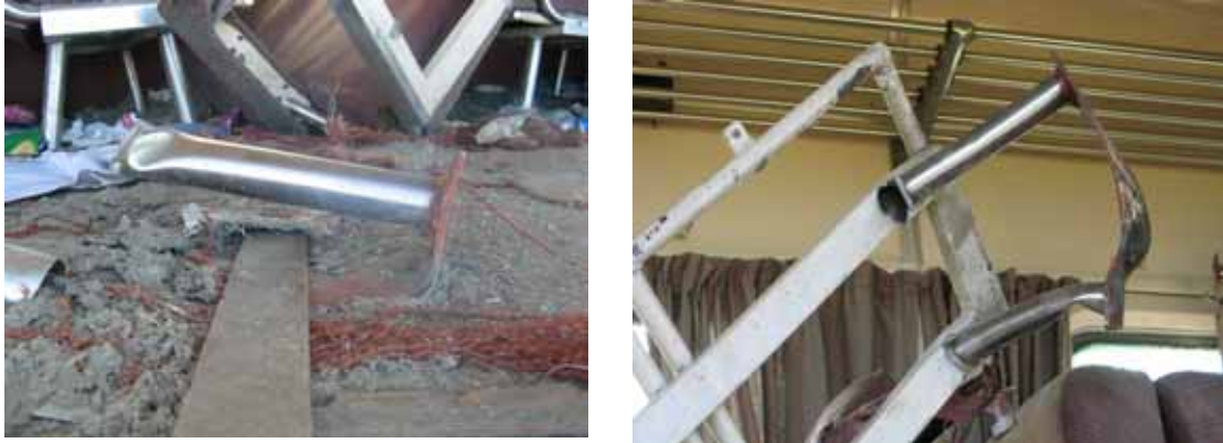
Figure 14. Bent base plate (left) and failure of upright to frame connection (right)
