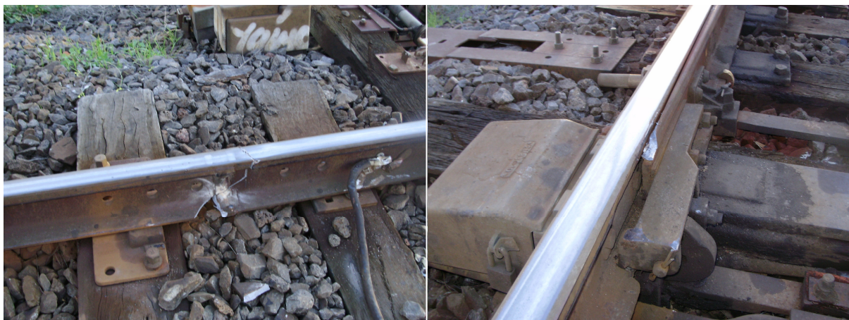
Figure 7 - Rail and Points damage
