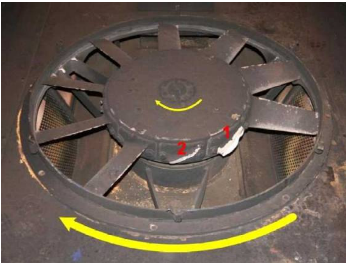
Figure 3 - Damaged fan assembly, showing direction of rotation of fan and frame
