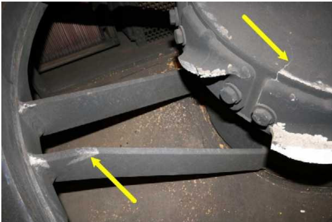
Figure 4 - Deformation of fan frame support arm and cracking of hub
