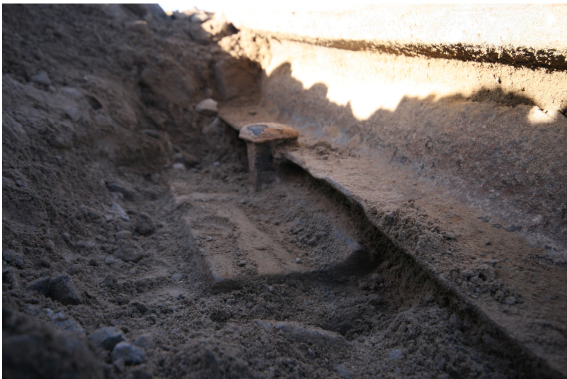
Figure 7 – Gap between sleeper support and rail at the Up end of the fracture
