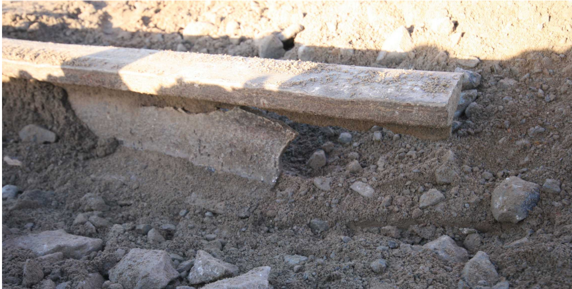
Figure 6 – Up end of fracture, in-situ (note continuation of horizontal web fracture)
