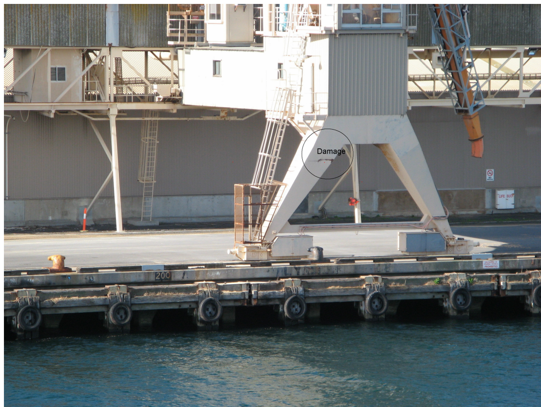
Figure 6. Damage to grain loader foot.
