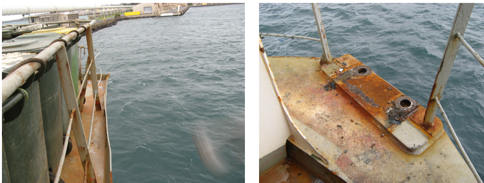
Figure 3. Damage to MV Portland.
