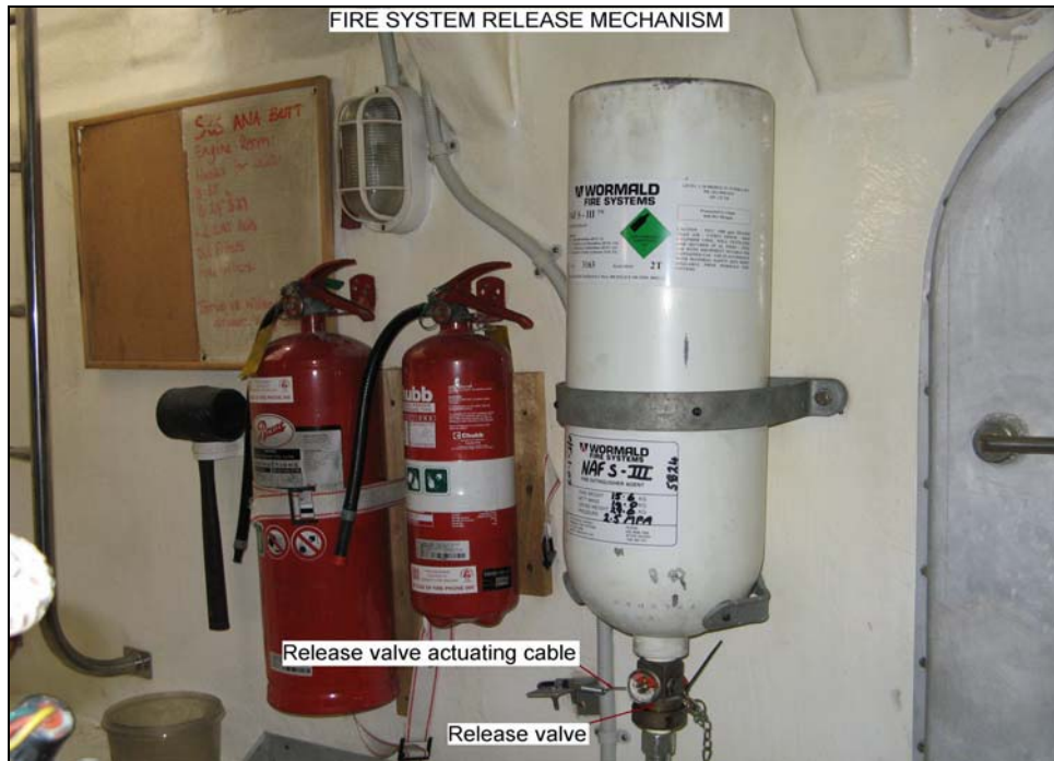
Figure 5 - Fire system release cable & valve
