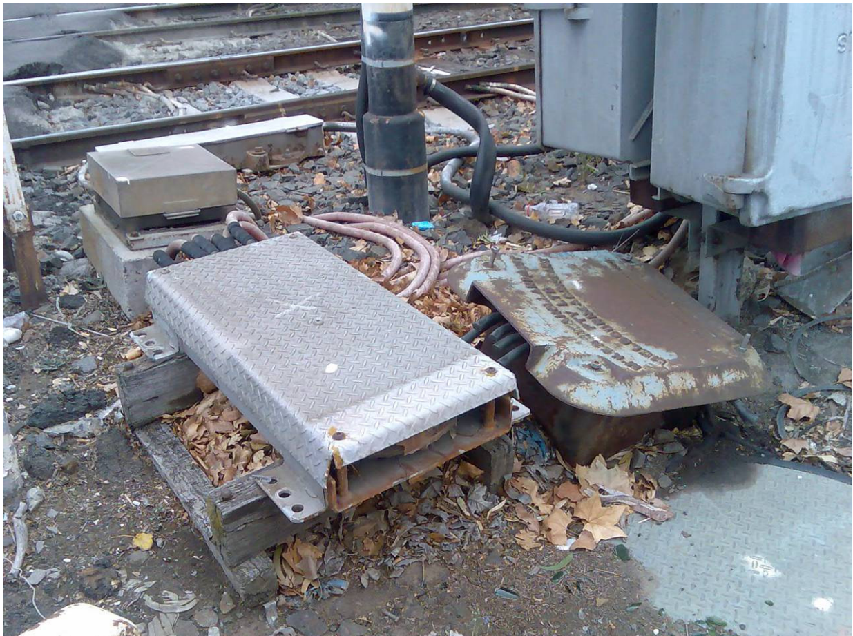
Figure 12 New impedance bond installation on original timber mounting at Kensington. The old impedance bond lies, discarded and disconnected, on the right.
