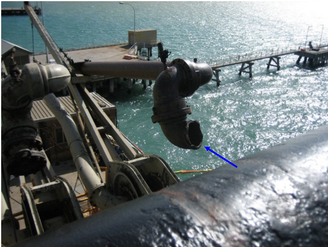
Figure 3 – Fractured shore cargo arm as seen from the vessel
