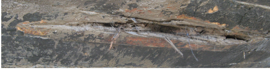
Fig 3: Close up of damage
