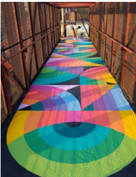
A colourful and playful approach to the resurfacing of Jersey City pedestrian bridge.
