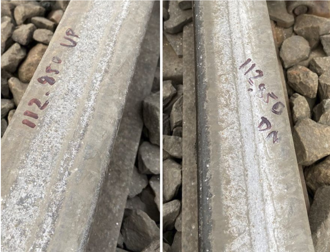
Figure 15: Rail surface condition at 112.850 km chainage, about 1.1 km from station stop
