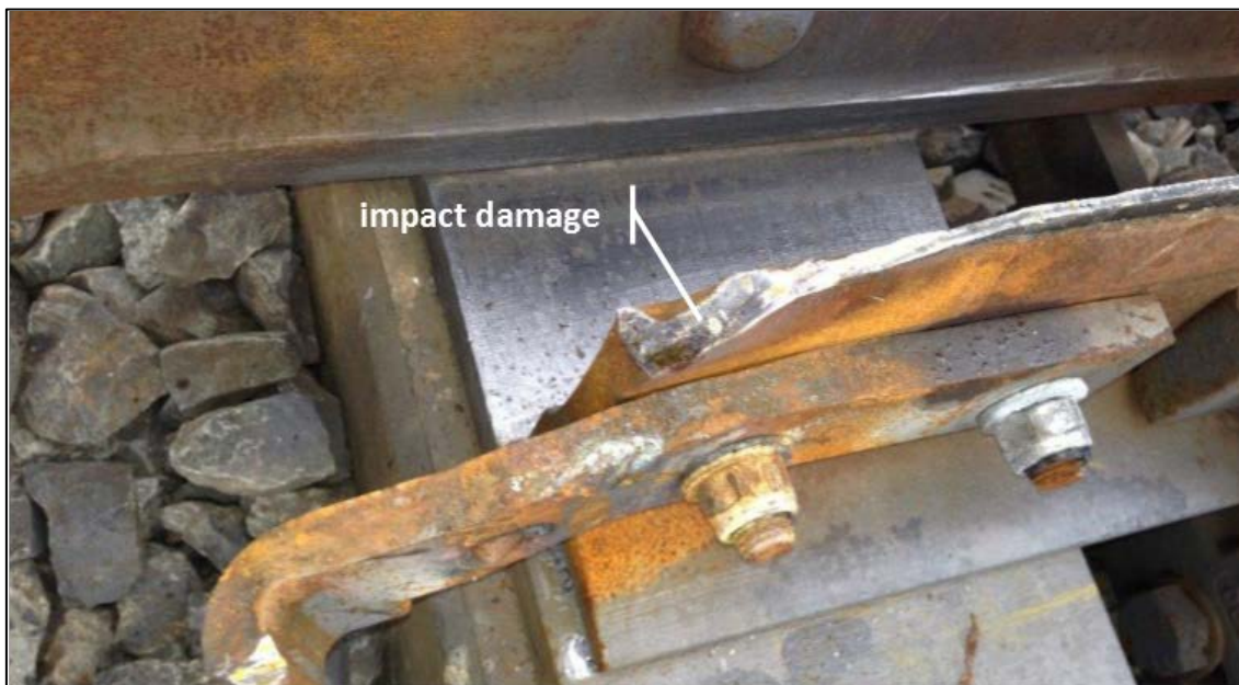
Figure 8: Impacted toe of the point blade at turnout 601
