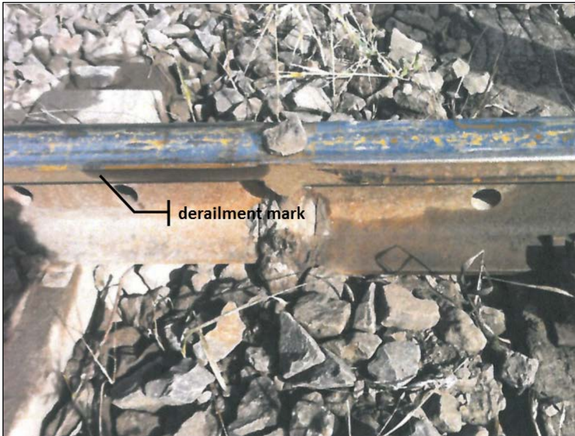
Figure 11: Photograph from the 11 September 2013 derailment, showing marks on the rail gauge face consistent with a left hand wheel dropping inside the common rail
