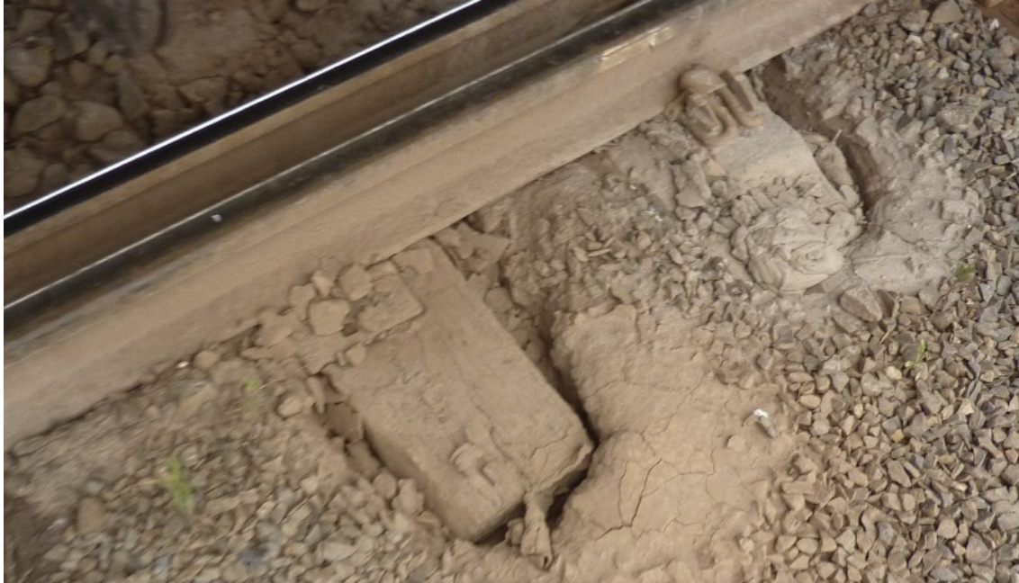
Figure 6: Track pumping at location of derailment
