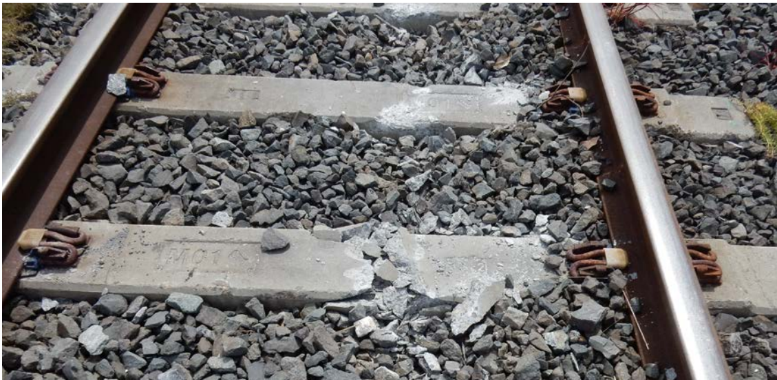
Figure 4: Typical damage to concrete sleepers within the crossing loop
