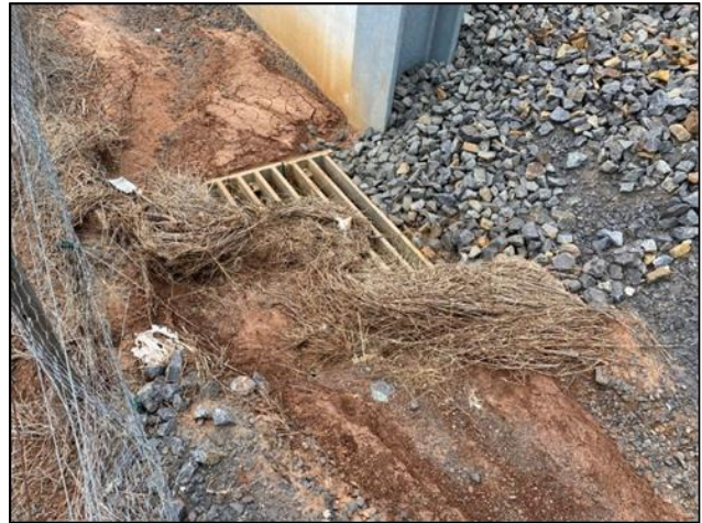
Plate 24. V/Line drain opposite the offset site fence line (southern boundary) blocked up with debris (Ecology and Heritage Partners 16/11/2021).
