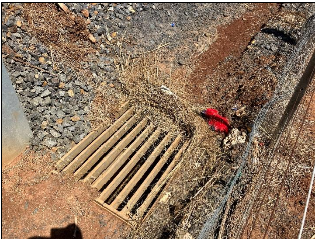
Plate 25. V/Line drain opposite the offset site fence line (southern boundary) relatively clear (Ecology and Heritage Partners 9/02/2023).
