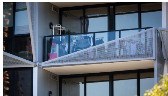
Balcony clutter increases ignition risk
