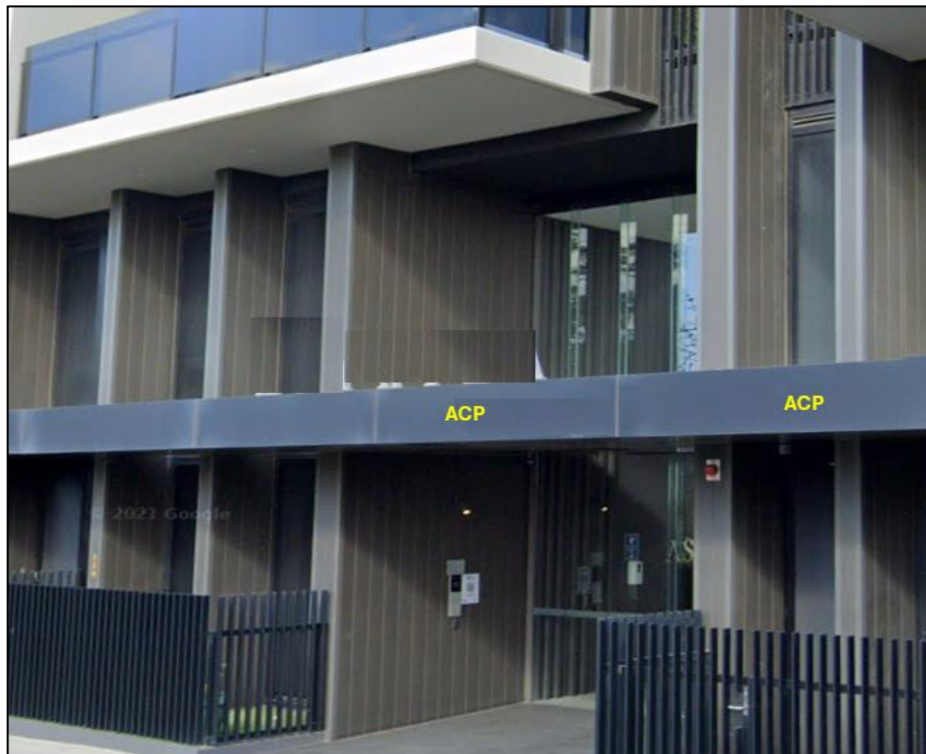
Figure 20: ACP canopy (soffit panels and fascia), sprinkler protection to SOUs no protection to exit.
