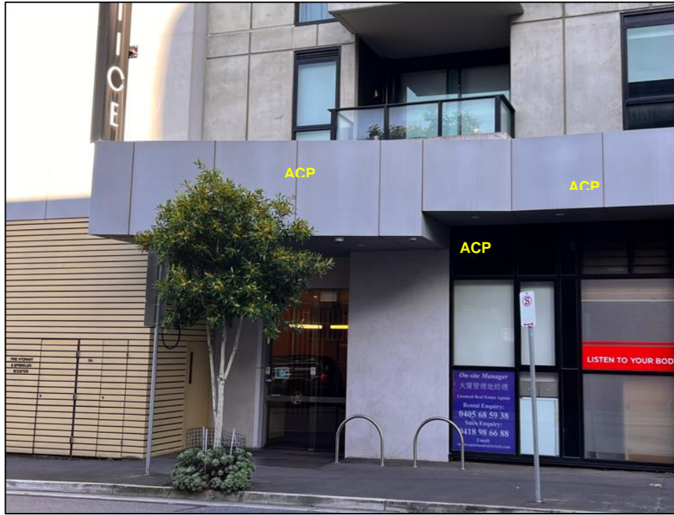
Figure 22: ACP to canopy (fascia and soffit panels) no protection from sprinklers.
