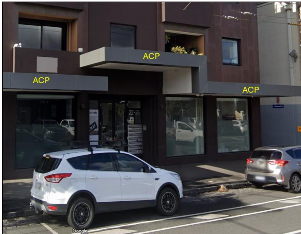
Figure 16: ACP cladding to fascia panels on canopy. Non-sprinklered building/exit.
