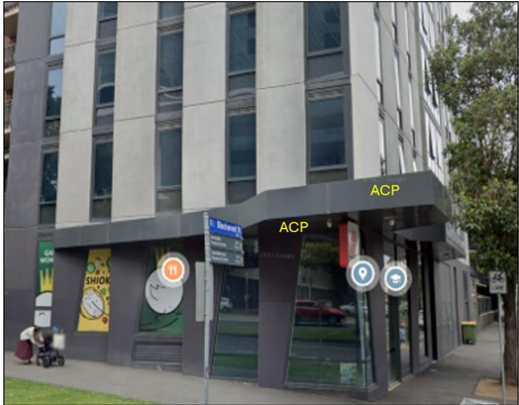
Figure 18: ACP panels to soffit and fascia of canopy. SOU and canopy is sprinkler protected.
