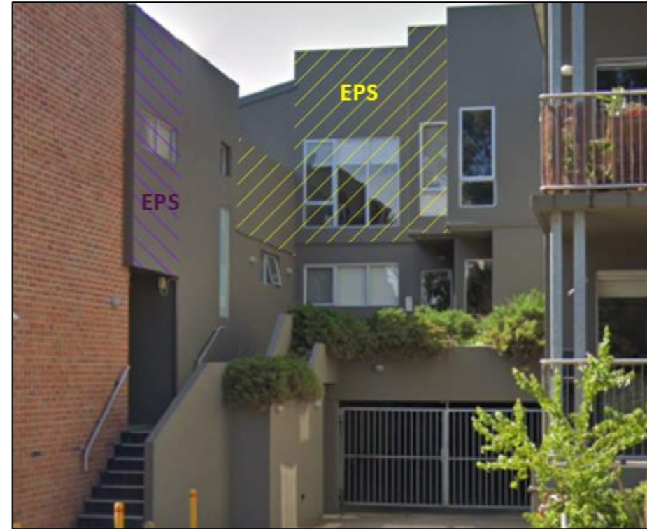
Figure 31: EPS cladding to the walls above the exit and the egress path from the exit – no sprinkler protection to SOUs or exit.
