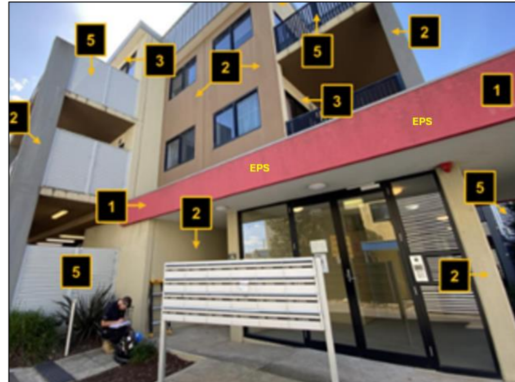
Figure 29: EPS used on the fascia of the canopy around the exit lobby.
