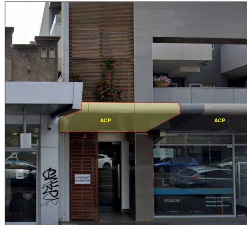
Figure 21: ACP to awning (fascia and soffit panels). No sprinkler protection to SOU or exit.
