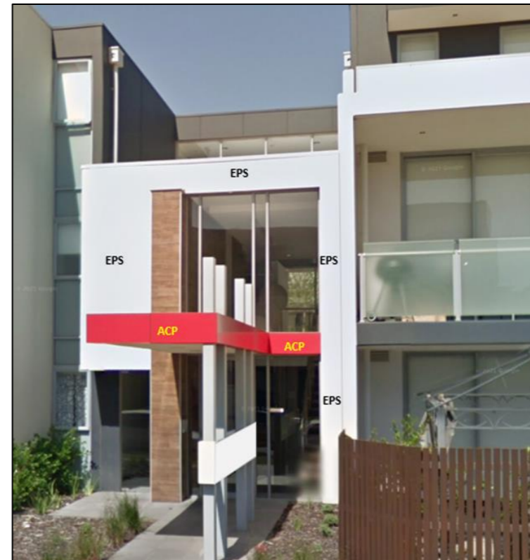
Figure 33: Exit has EPS that extend to the garden bed on the side of the exit. The exit canopy has ACP fascia lining with non-combustible soffit.
