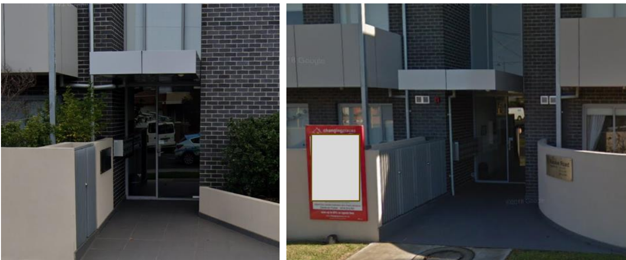
Figure 5: ACP located to the fascia of the canopies only. Soffits are non-combustible and void of likely ignition sources
