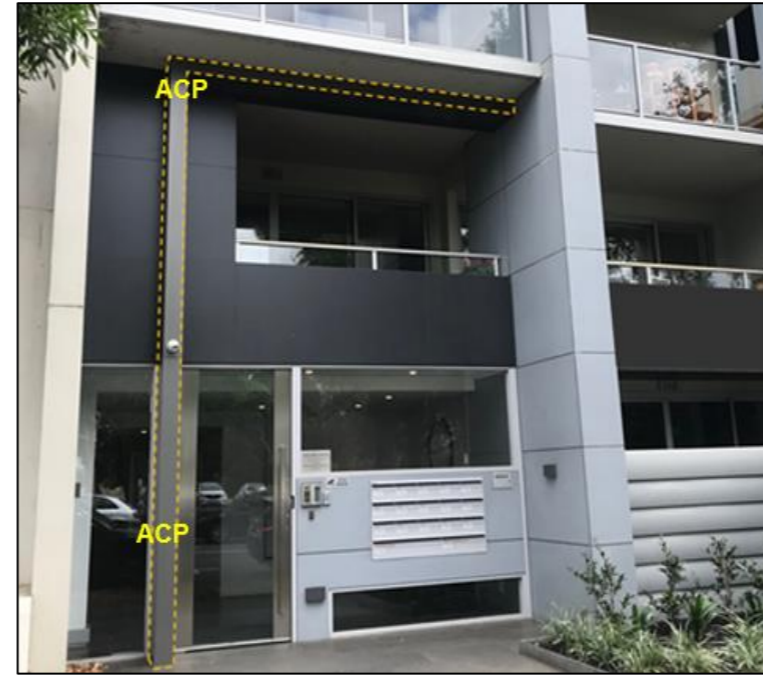
Figure 47: ACP element to the left side of the singular exit on the building. Sprinkler protection to SOUs.
