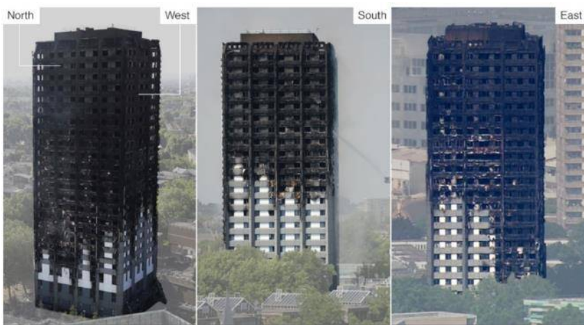
Figure 54. Grenfell Tower post fire damage (image from BBC News [64] )
