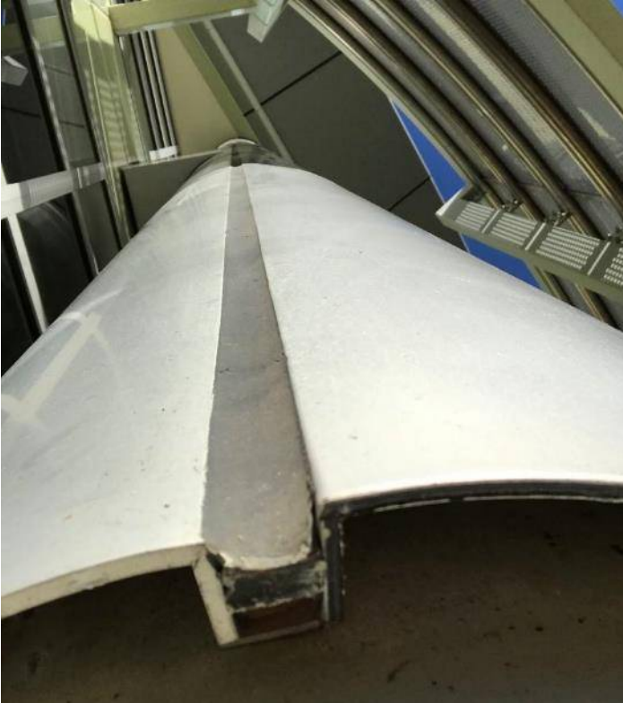
Figure 16. ACP with same colour external facing but different cores used on same building (Photo by CSIRO)
