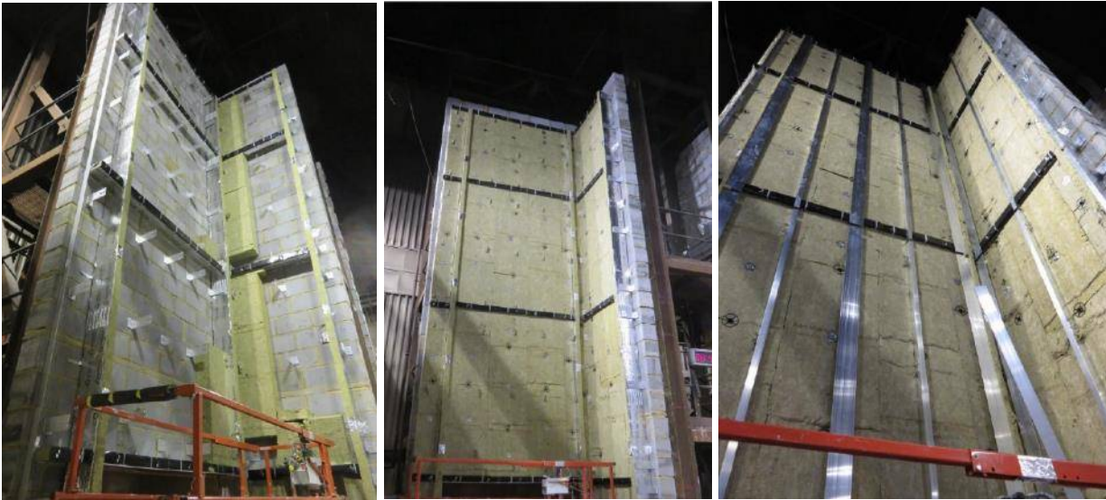
Figure 45 Left – Horizontal and vertical cavity barrier installed through entire depth and aluminium cladding support brackets bolted to masonry wall (MW insulation being installed to wing wall), Centre – cavity barriers and MW insulation installed, Right – Aluminium railing sub structure installed (all photos taken from BRE test report [51] )
