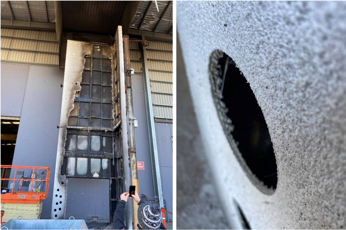
Figure 13. Post-test wall system showing render thickness hole saw samples. Right photo shows close up hole saw sample on left side of combustion chamber with EPS behind completely melted/burnt away.
