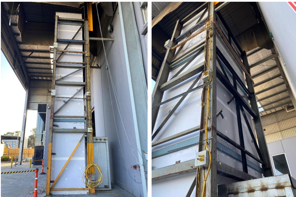
Figure 10. Post-test wall system non-fire exposed side. Wing wall (left), Main wall (right)
