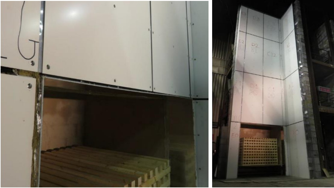
Figure 15. Left – Aluminium window pod, combustion chamber and ACP joints and fixing detail. Right – complete façade system prior to test (all photos taken from BRE Test report
