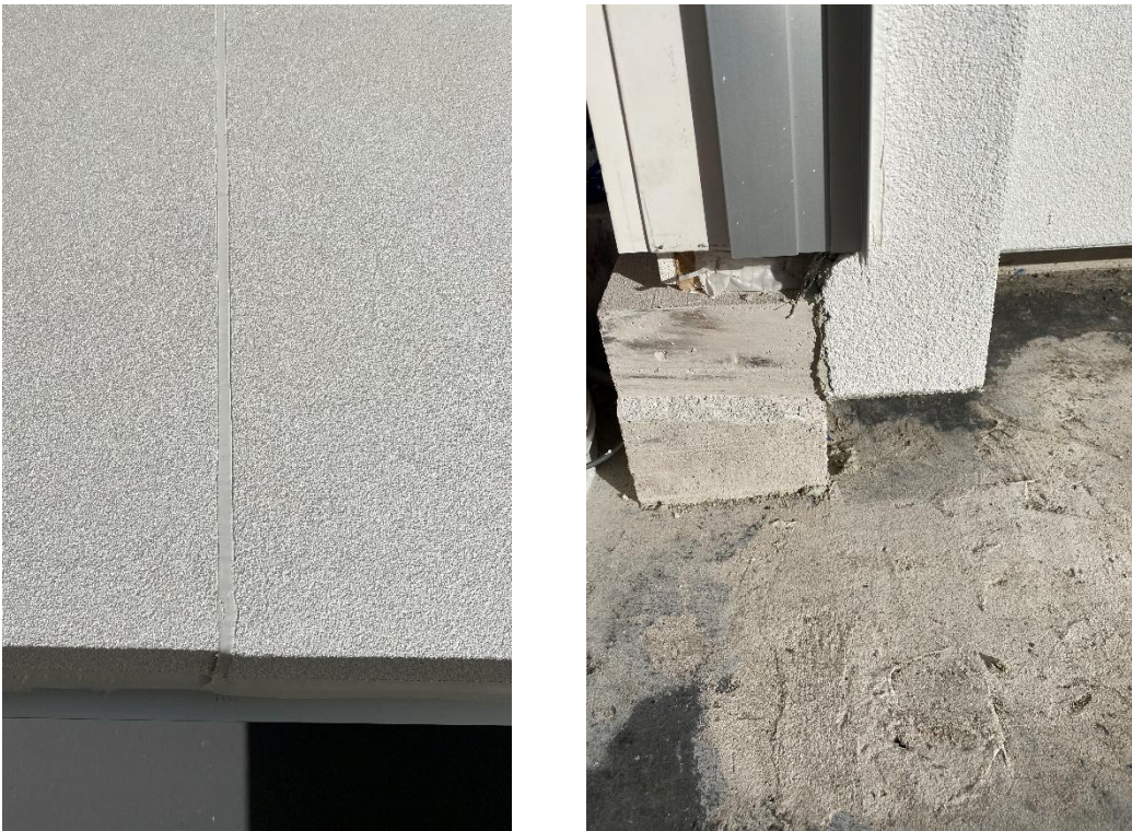
Figure 5. Vertical construction joint (left) and edge of combustion chamber (right) showing simulated timber window reveal and Hebel block simulating slab edge) during CSIRO inspection of completed construction at Warringtonfire.
