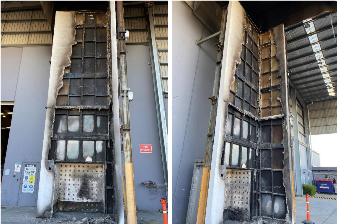
Figure 11. Post-test wall system with all regions of heavily heat affected render removed showing EPS behind melted/burnt away
