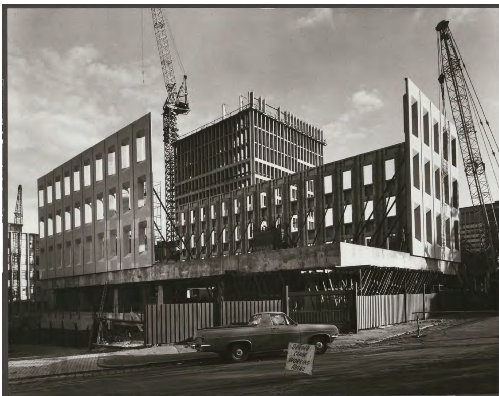
Figure 60: Sievers, W., & Yuncken Freeman Architects. (1967). Lifting and Fitting Pre-cast Concrete Panels, Government Laboratories Block, State Government Offices, Macarthur Street, East Melbourne, H2000.195/336, Pictures Collection, State Library of Victoria. CLPC products from the Employment Precinct have been used to build Melbourne.
