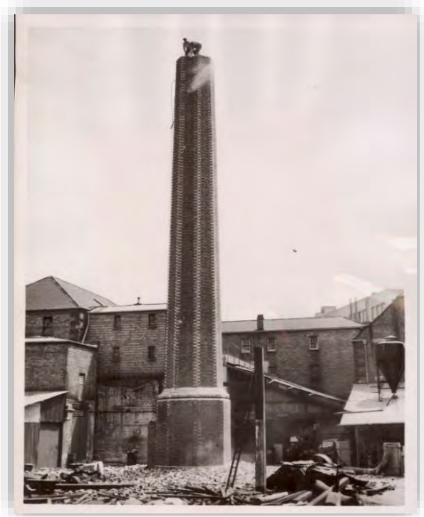
Figure 12: Hansford, P & Argus (1954) Chimney being demolished, H2002.199/672, Pictures Collection, State Library of Victoria
