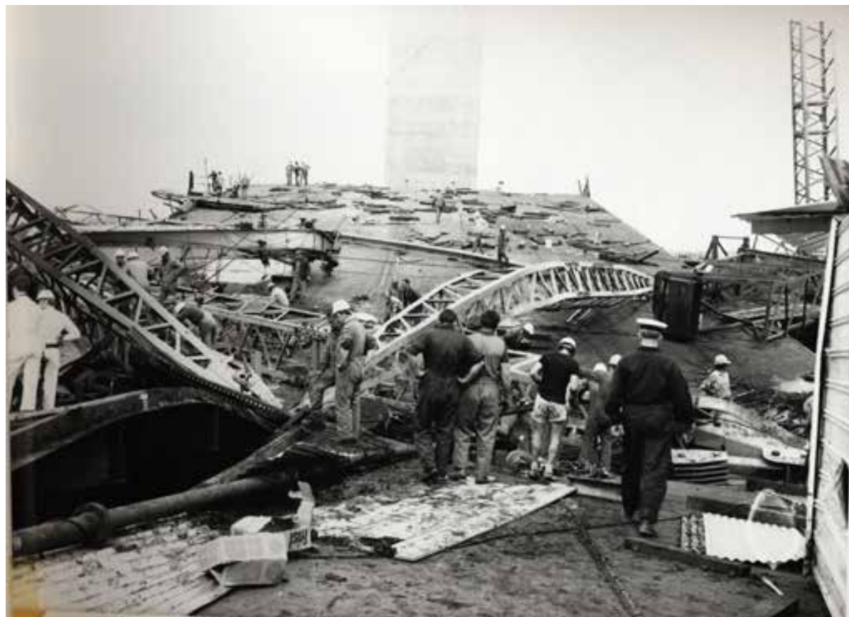
Figure 24: Collapse of the West Gate Bridge in 1970, during construction (source: PROV)
