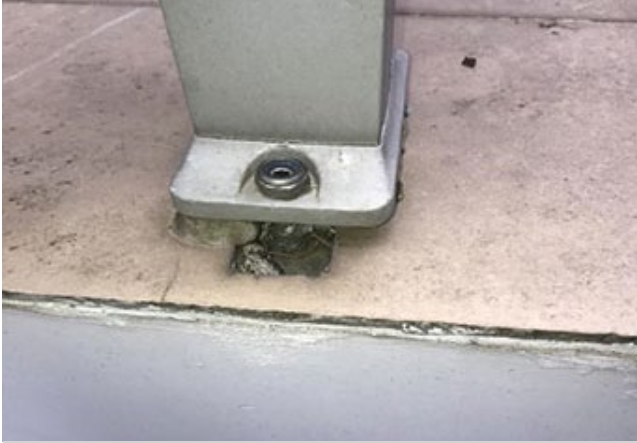
Improper water proofing around balustrade fixing providing areas for water ingress to structural elements.
