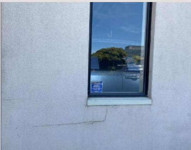
Cracking along blockwork joints.
