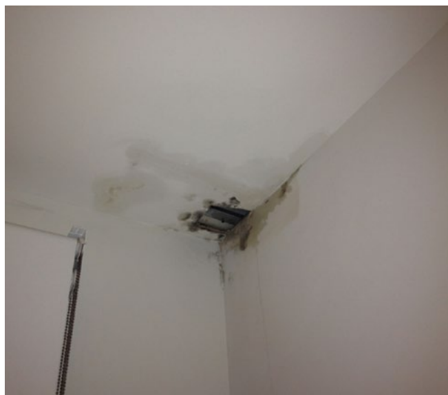
Moisture seeping through plaster walls.
