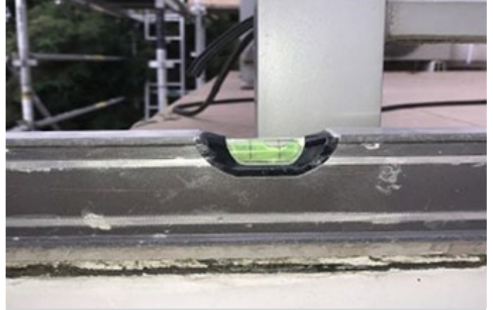
Balcony falling steeply away at edge.
