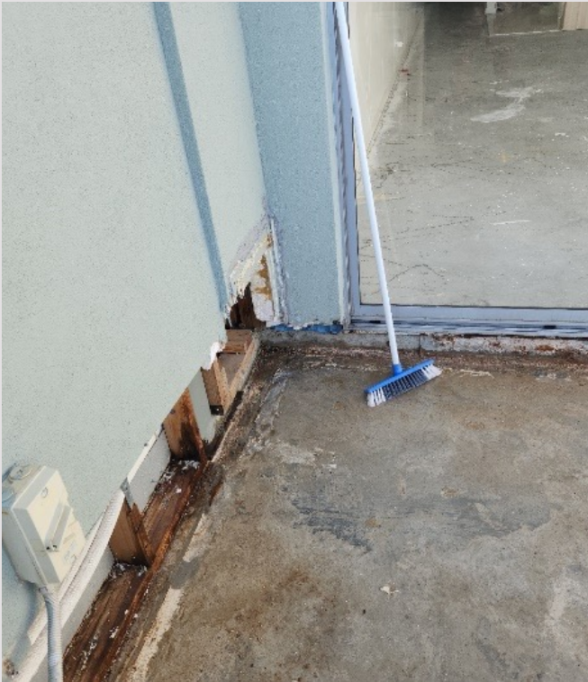
Rotten framework caused by water ingress.
