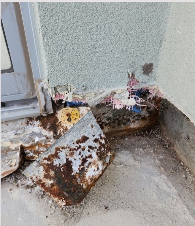
Corroded steel frames caused by water leakage.
