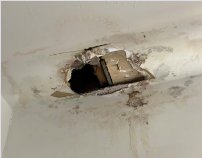
Mould and staining on apartment ceiling.
