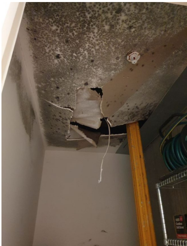
Figure 7. This apartment's ceiling has collapsed after years of water collected from the balcony above it
