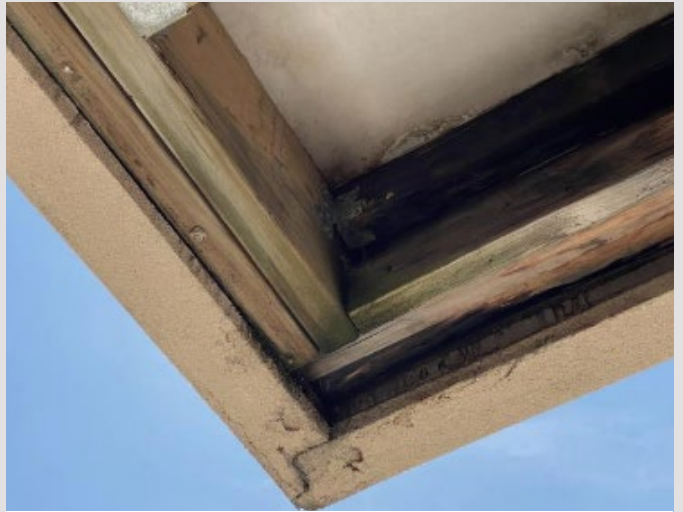
Deterioration of timber balcony.
